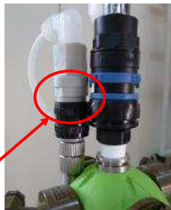
Bad: There is a gap → Not firmly connected
