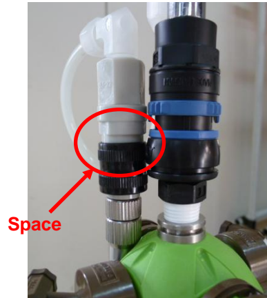
Bad: There is a space → Not firmly connected
