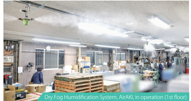
Dry Fog Humidification System, AirAKI, in operation (1st floor)
