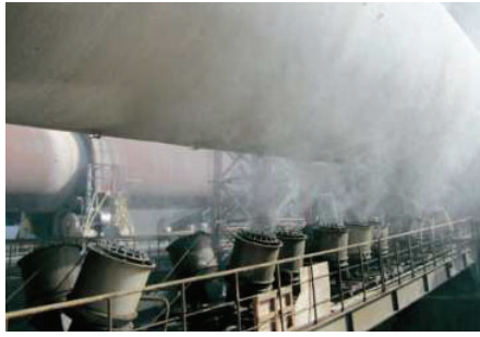
Industrial cooling system
