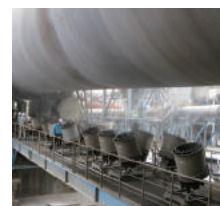
Kiln cooling system
